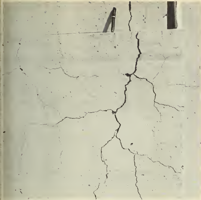
FIGURE 3. Cracks in pier, Sixth Street Bridge, Los Angeles.
